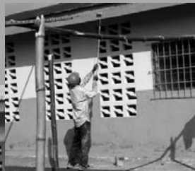
▲ In the congregation of Foya Kpadonin, the brothers and sisters were very pleased to contribute to the preservation of their church building.
